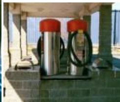
Hwy 501 Covered Vacuum
